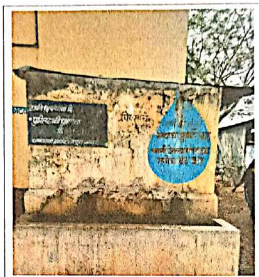
Drinking Water Tank
